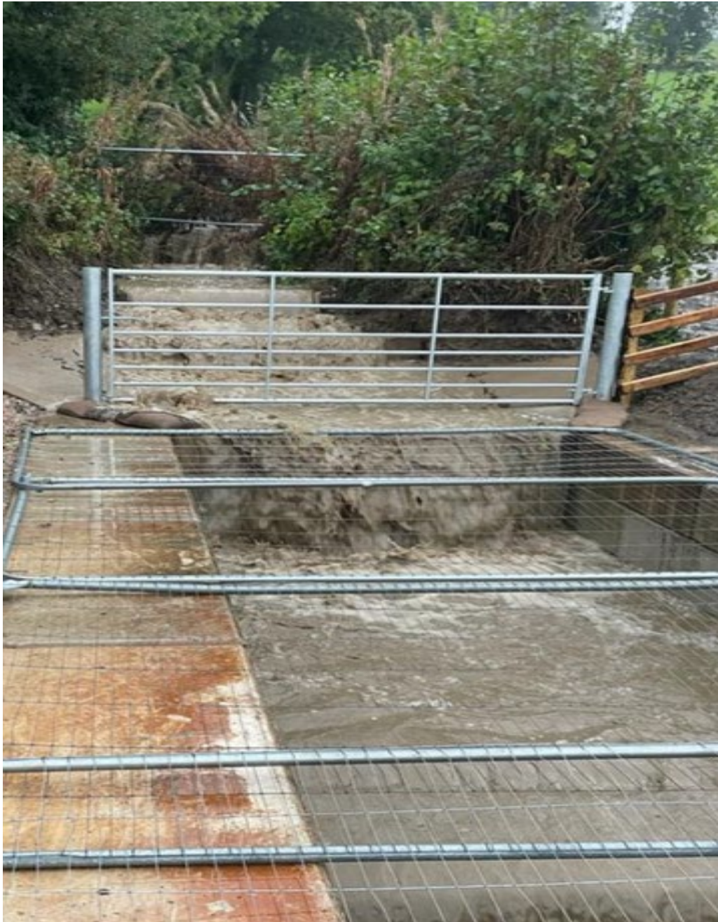
Photo 13: New culvert structure at Nantglyn Village during Storm Babet
