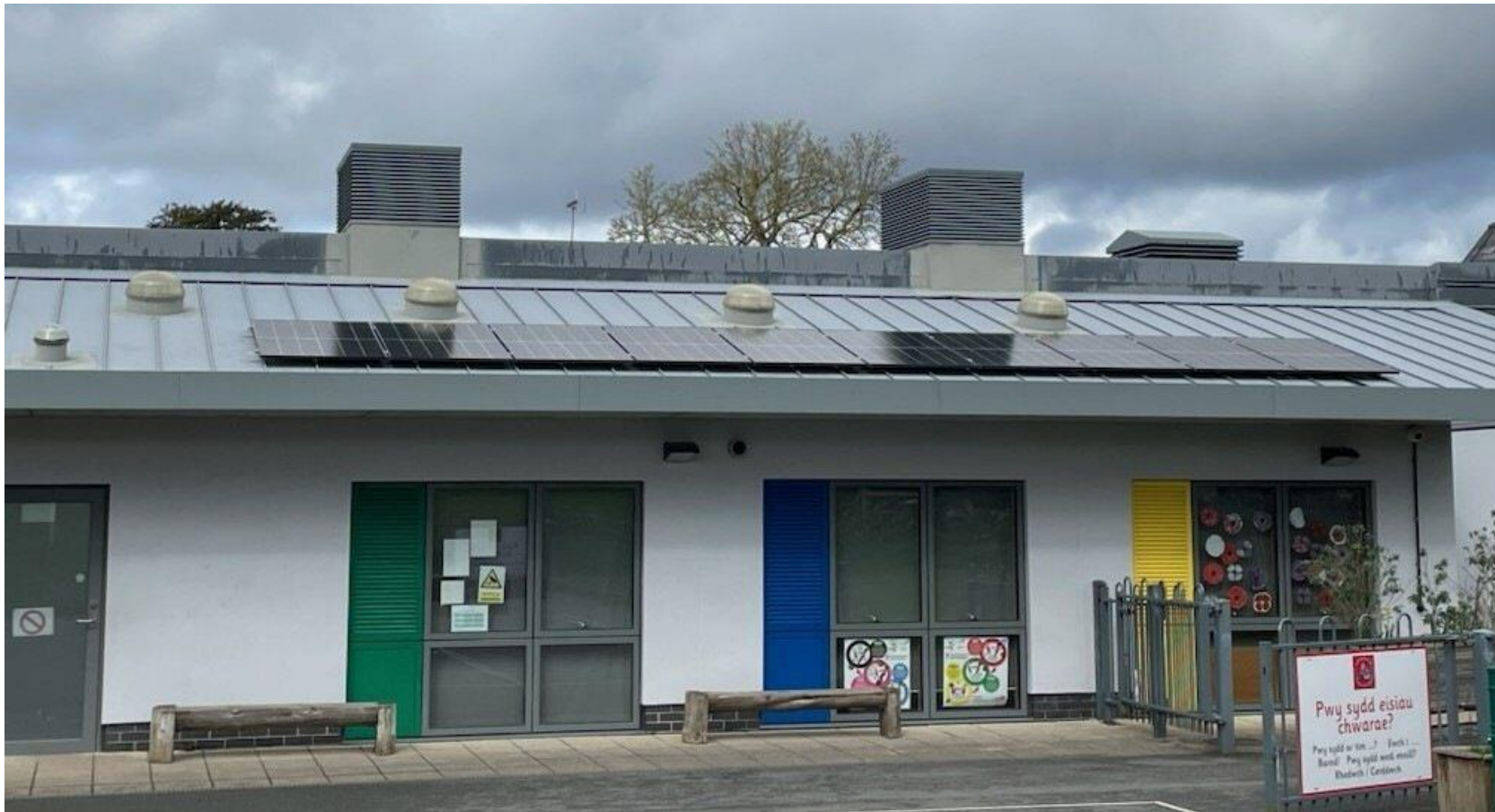
Figure 3.0.1 : Rooftop solar PV at Ysgol Dyffryn Iâl, Llandegla, Denbighshire
