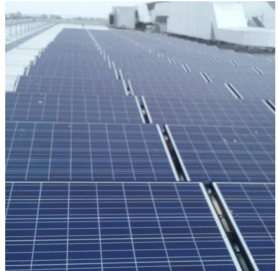
Figure 2.0.5: Rooftop solar PV panels
