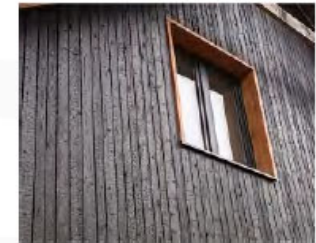
Charred timber to inset balcony
