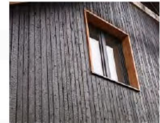
Charred timber to inset balcony
