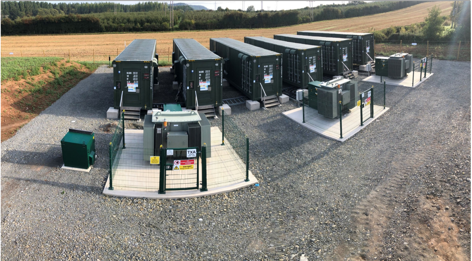
Example utility scale battery storage units ( https://anesco.co.uk/utility-scale-battery-storage/ )
