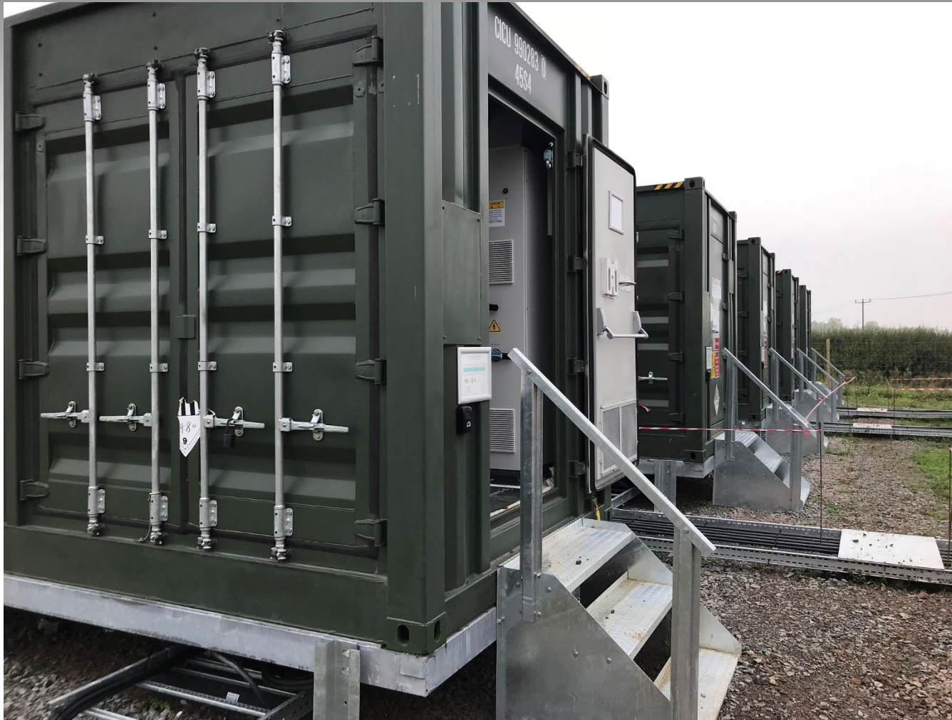
Clay Hill solar farm
